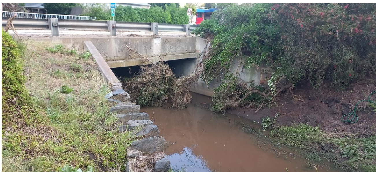
Figure 2-4: Tree branch against the Goolwa Road culverts
